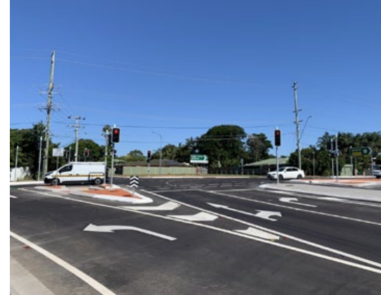
The new Jellicoe St/Station Rd, Loganlea intersection pictured from the Logan Motorway exit
